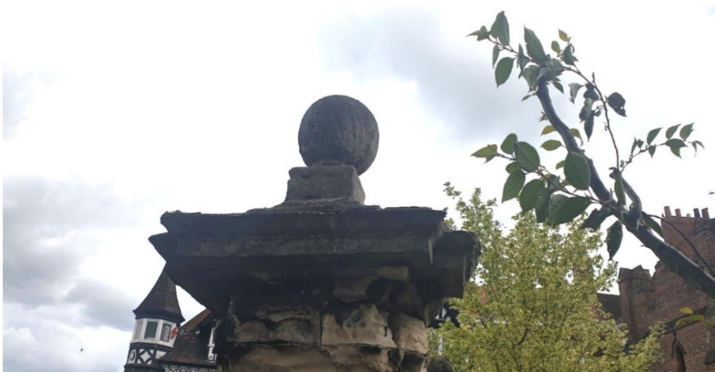
Picture of ball after roadworks and before restoration with minimum intervention as required by the conservation officer.
